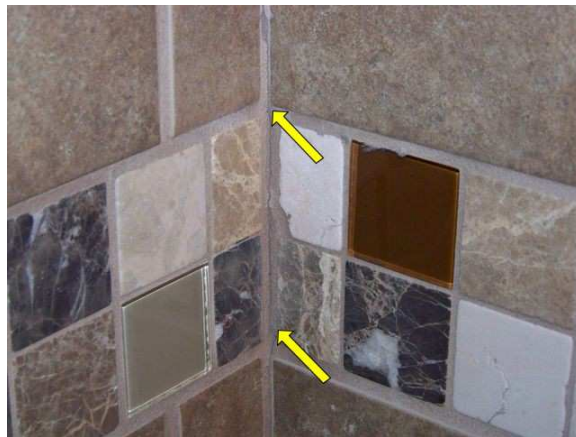
Caulking or grout in need of repair
