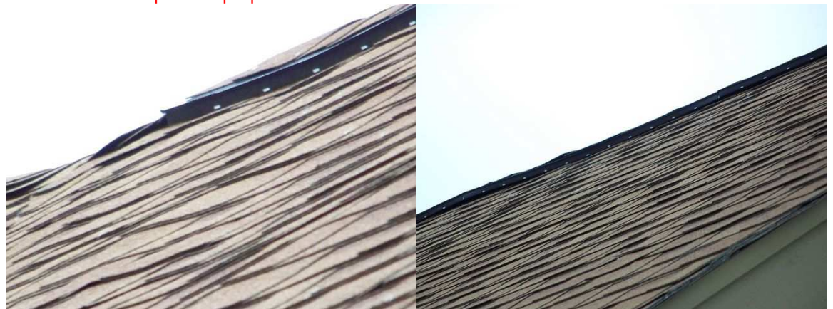
It appears the ridge caps do not completely cover the ridge vents
