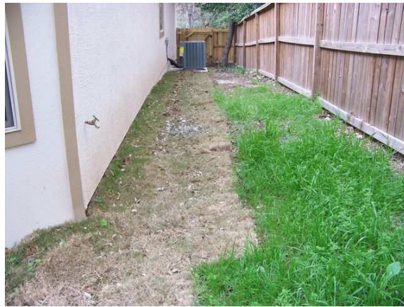
Soil shall be graded to drain surface water away from the foundation. The grade shall fall
