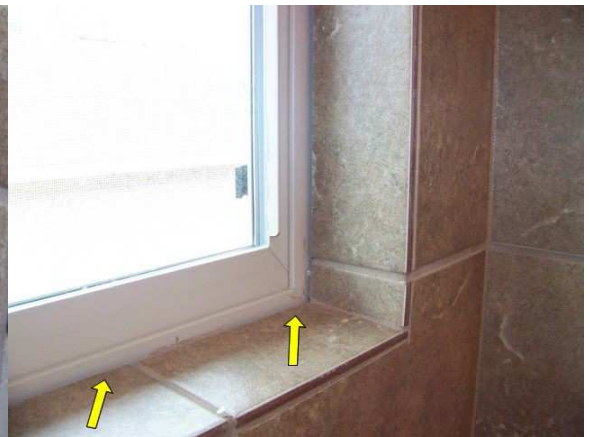
Enclosure needs to be sealed
