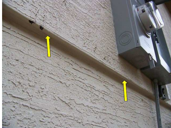
No weep screed installed
