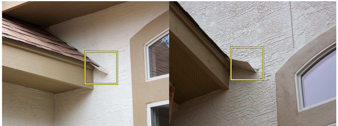
No kick out flashing installed
