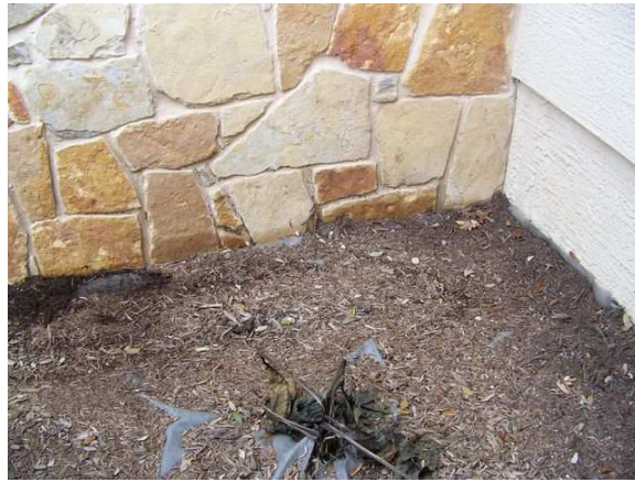
Inadequate grading clearance to exterior wall surface
