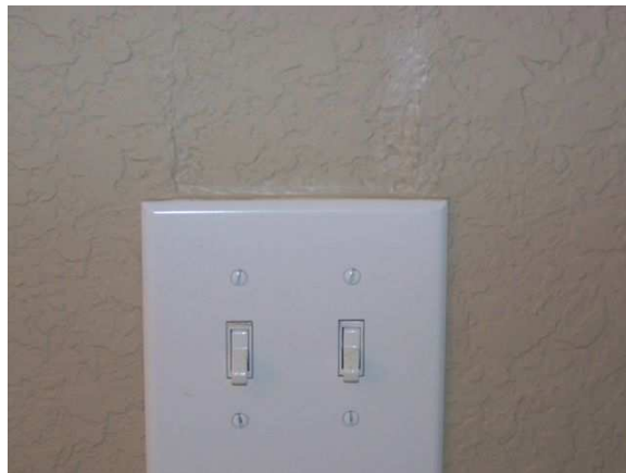
Patch above light switch visible
