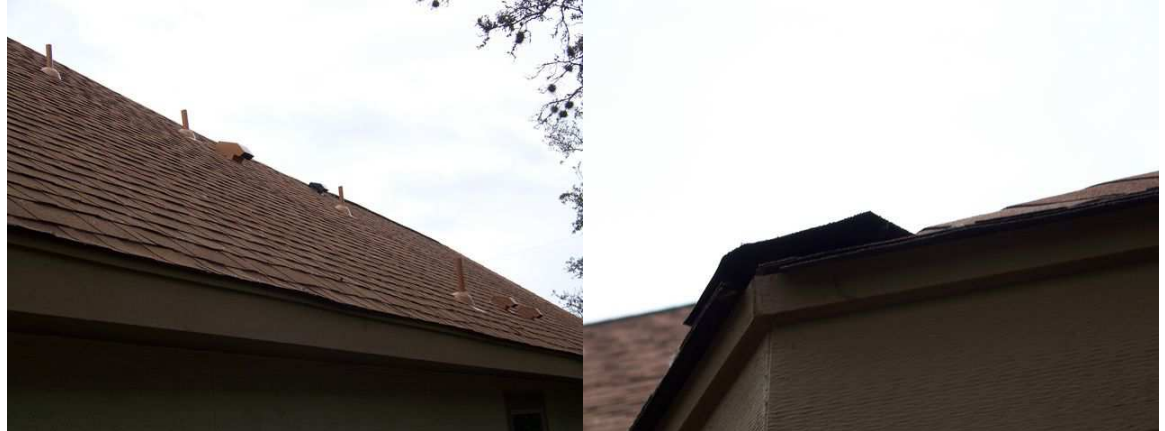
Roof decking deflection and/or sagging
