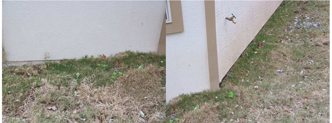
Inadequate grading clearance to exterior wall surface
