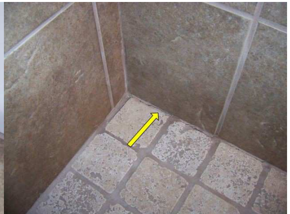
Caulking or grout in need of repair
